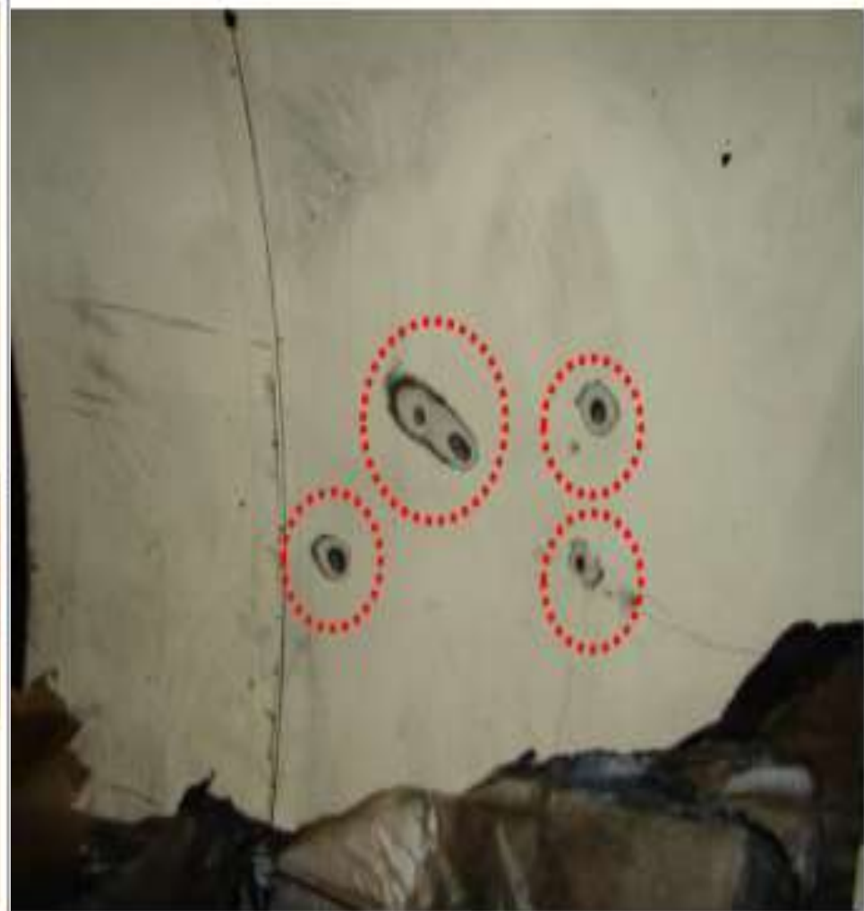
Arcing marks on the inner surface of bushing housing
